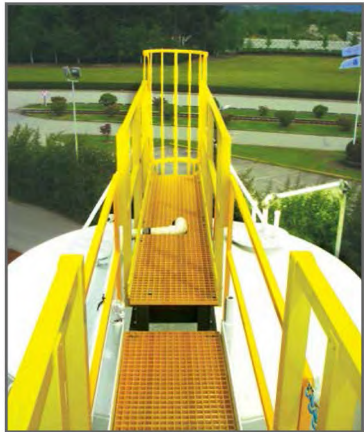
ZeAllgrate's grating, railings and structure create walkways for worker access to multiple tanks.
