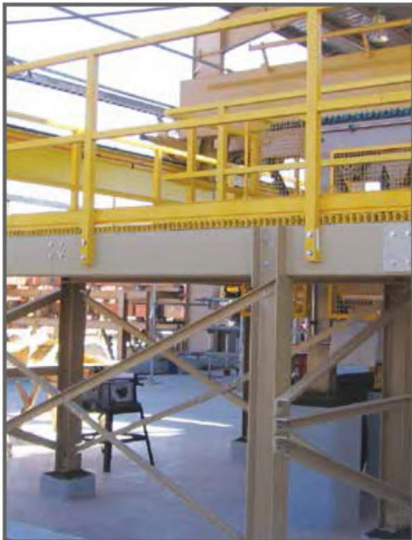
ZeAllgrate structural shapes and pultruded grating were used in this mining facility for their corrosion resistance.
